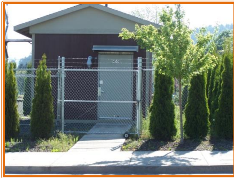
Telecom Hut located on South 6 th Street
