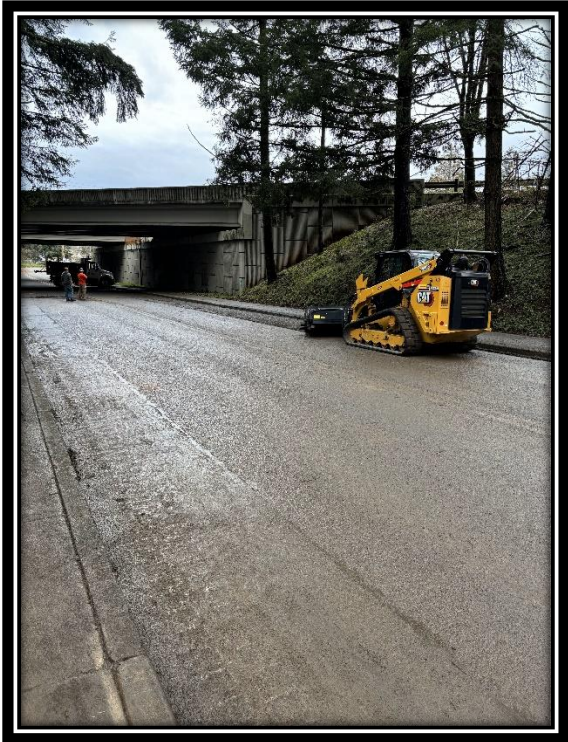
2024 Ice Storm Debris Removal from Streets
