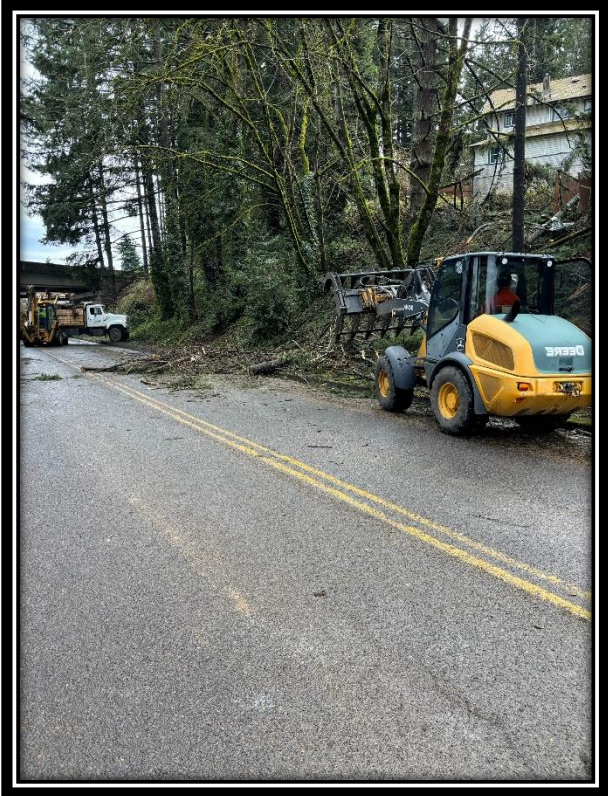
2024 Ice Storm Debris Removal from Streets
