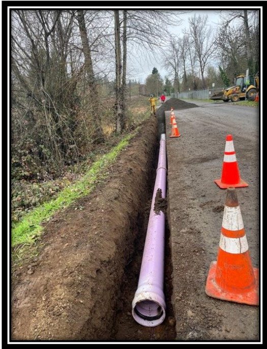
12" Water Treated Effluent Line
