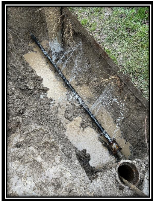
Leaking Water Mainline
