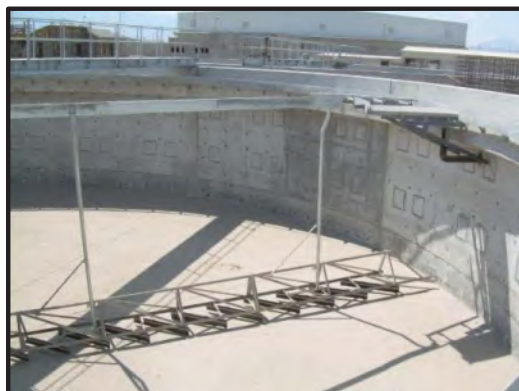
30.5M PRIMARY CLARIFIER – MEXICO
