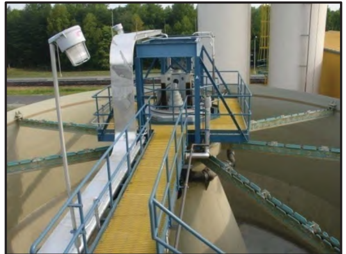
50' REACTOR CLARIFIER – NORTH CAROLINA, USA
