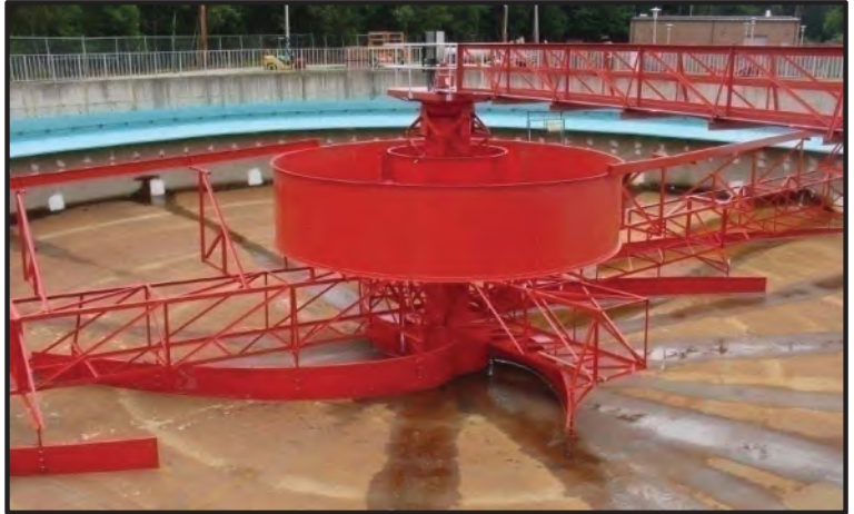
145' SECONDARY CLARIFIER – NEW HAMPSHIRE, USA
