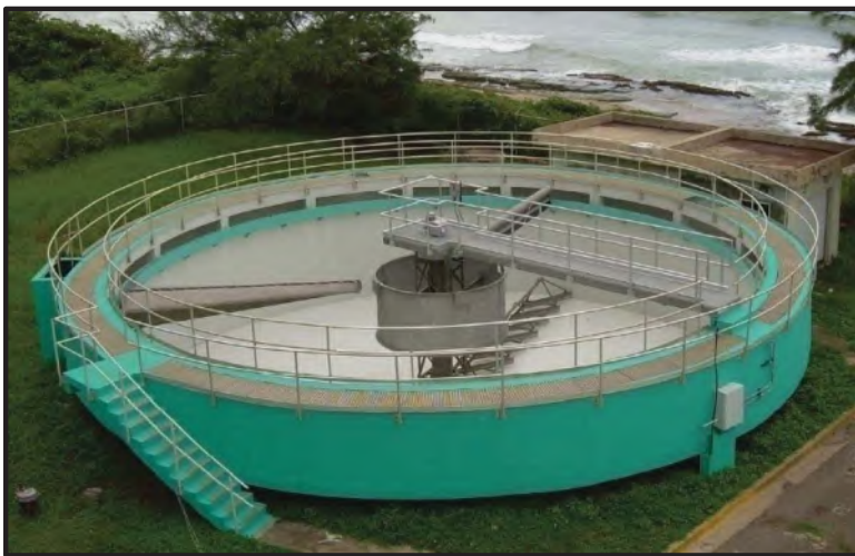
50' CLARIFIER – PUERTO RICO
